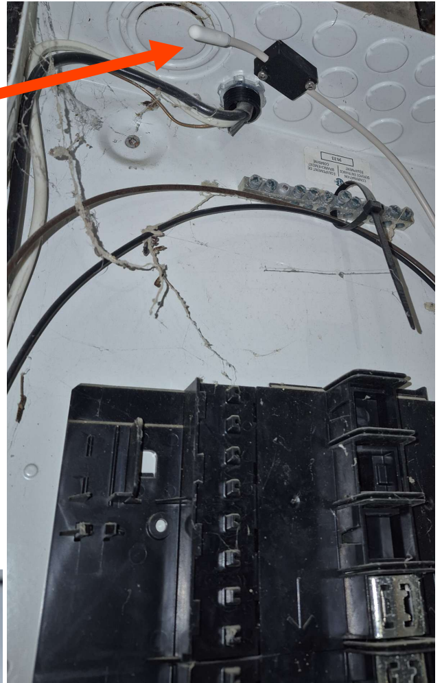
Fig 7, Panel Temp probe on highest breaker panel face
